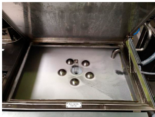
Example of oil separator suction unit
